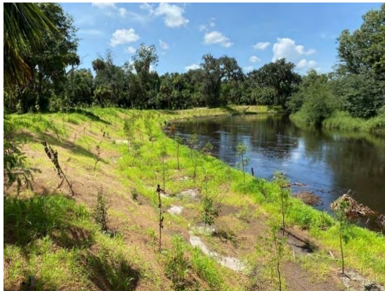
Figure 8. Field photos before (top), during (middle), and after (bottom) restoration at the 450-ft streambank on the Peace River near Zolfo Springs, FL.
